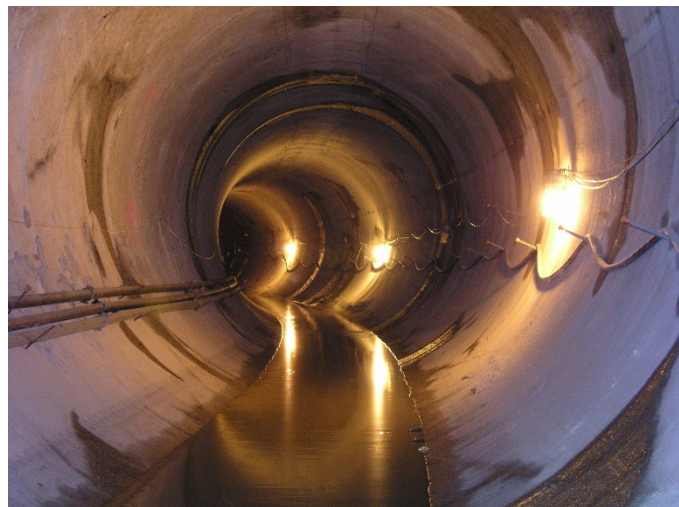
Figure 14. CSO tunnel (photo courtesy of the City of Fall River)
