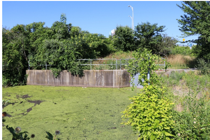
Figure 7. Plymouth Avenue intake structure
